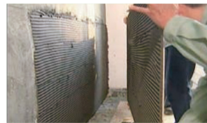
8, All notches on the substrate and porcelain panel shall parallel with each other
