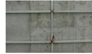
1, Install the main frame according to the overall design requirements for size distribution
